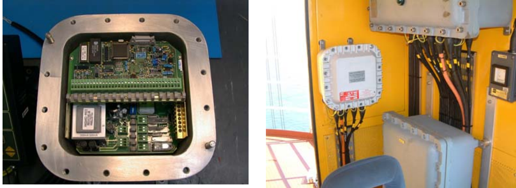
Typical installation of control unit inside the operator's cabin
